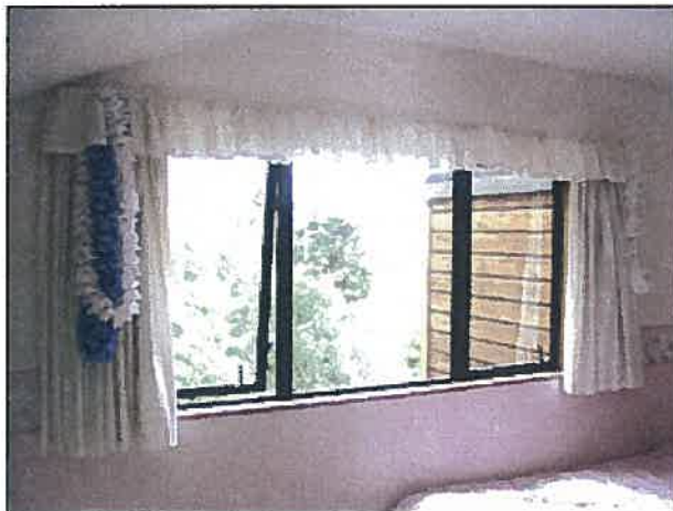
View of 'pushed-out' side wall to bedroom 4.
