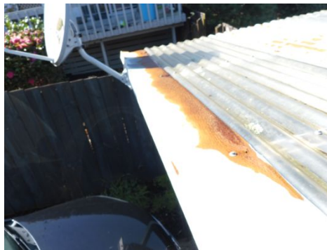
Surface corrosion present
