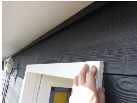
Missing head flashing
