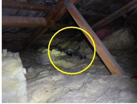
Dose not appear to be ducted
