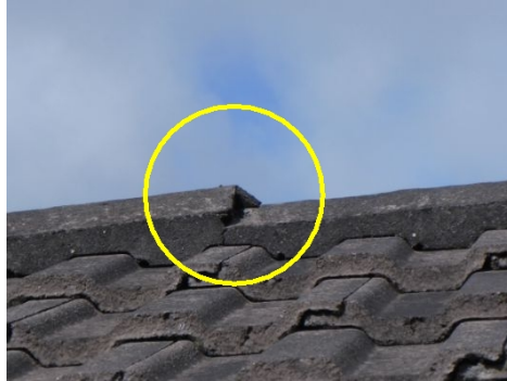
Cracked mortar present
