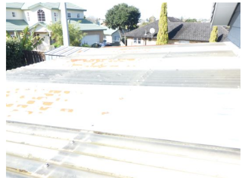
Surface corrosion present
