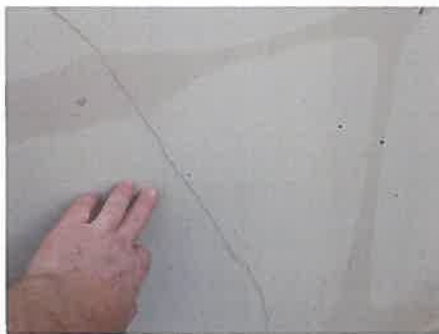
Some cracking present
