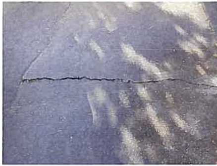
Cracked concrete present
