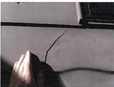
Cracked fiber cement
