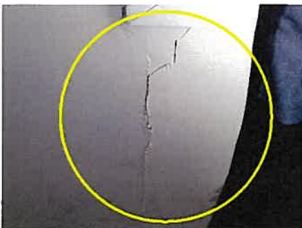
Damaged wall lining
