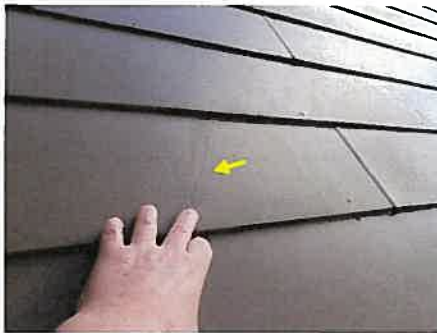
Cracked fiber cement
