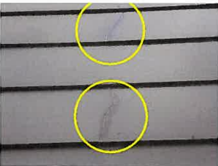
Cracked fiber cement
