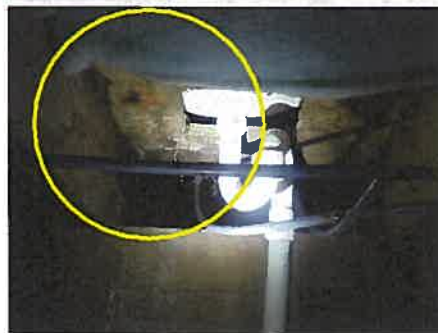
Moisture effected floor
