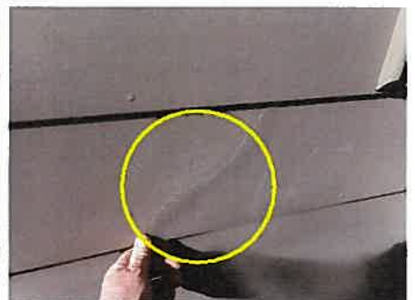
Cracked fiber cement
