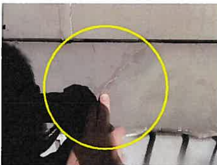
Cracked fiber cement
