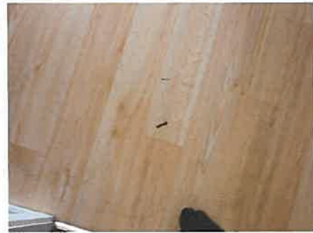
Some damage present
