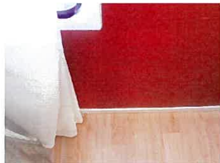
Damaged wall lining
