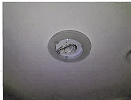
Missing light cover
